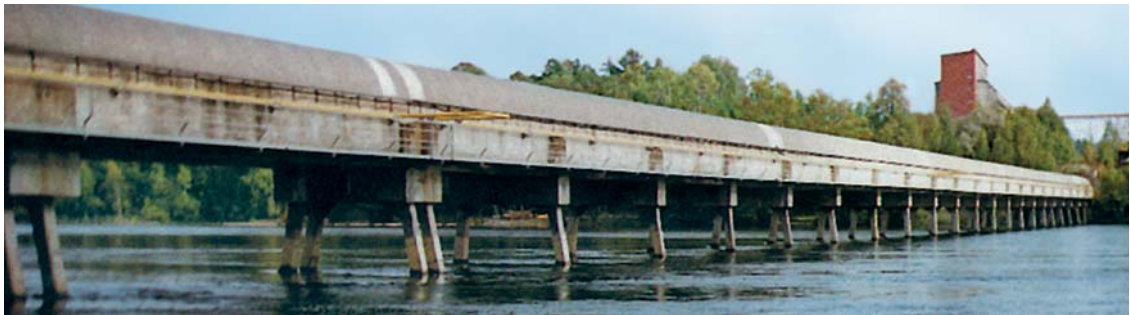
Sealing of a pipe running across a bridge in Scandinavia with AMEX ® -10 Internal Sealing System, temperature range: -30 °C to +25 °C.
