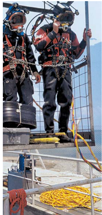
Installation of AMEX®-10 MONO Seal with divers in a flooded pipe system
